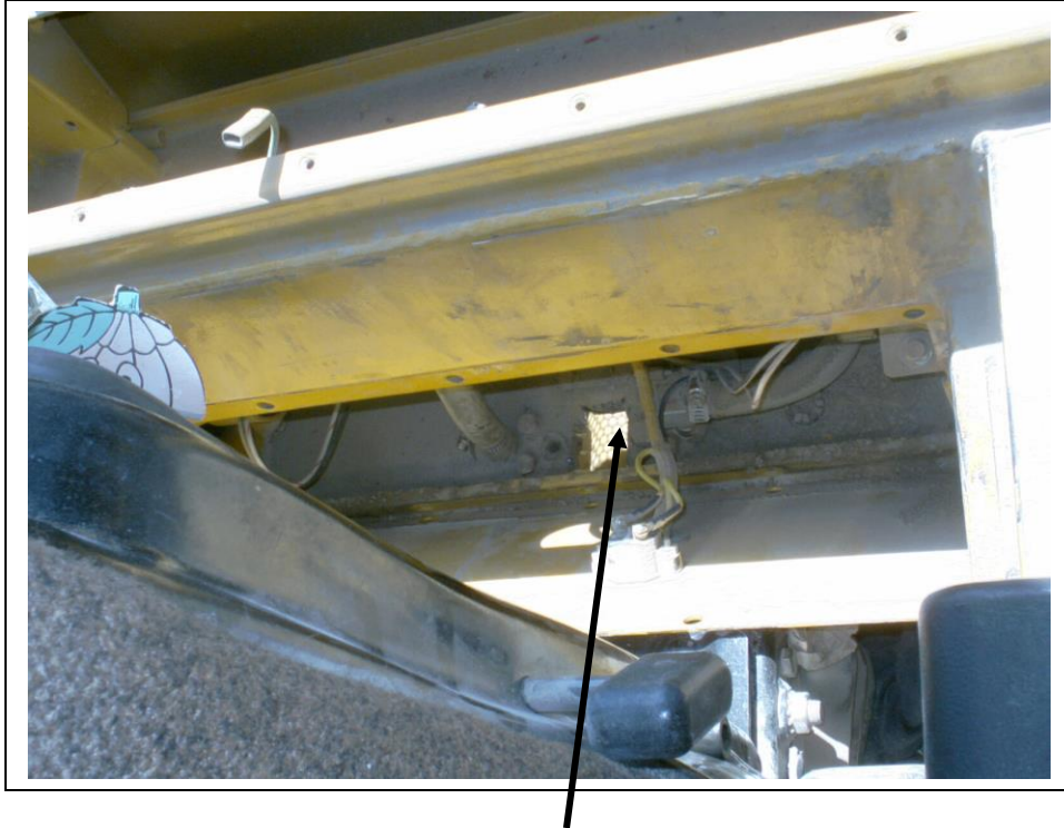
Drill, cut, chisel open this area to allow A/C hoses into the cab.
